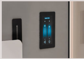
Air flow and lighting dimmer
